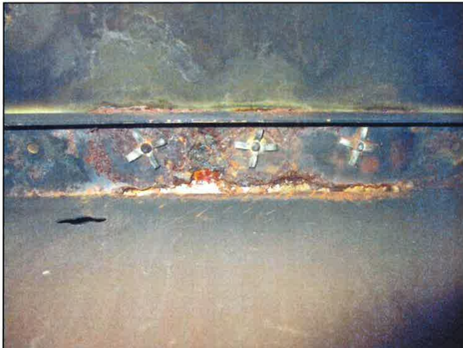
Photo 4: Localized section of severely corroded roof Z-purlin at interface of top flange and web View looking up.
