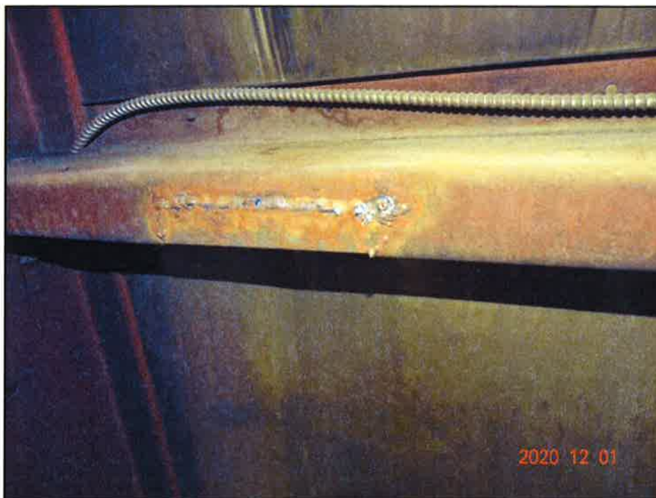
Photo 10: Coupon repair at wall girt with incomplete joint penetration weld and requires coating with zinc rich primer.
