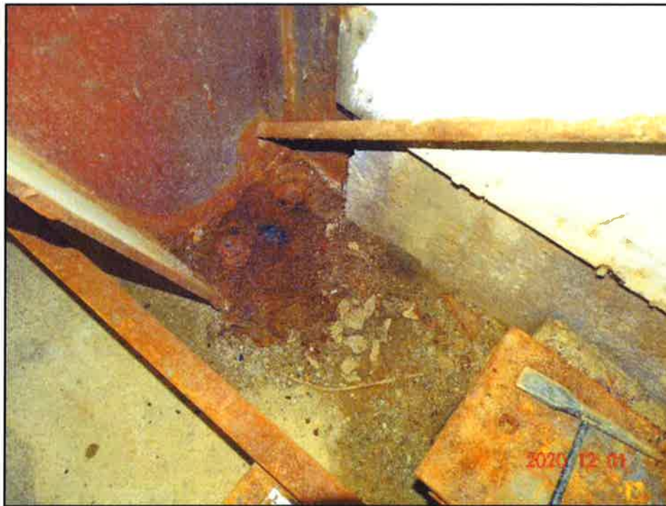
Photo 6: One of two Severely corroded rigid frame column base plate and anchor bolts along east wall
