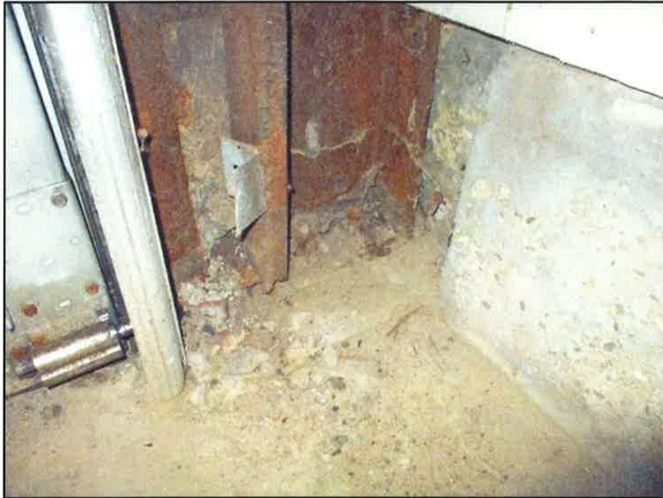
Photo 3: Localized severe section loss due to corrosion of bottom of exterior north wall framing end column.
