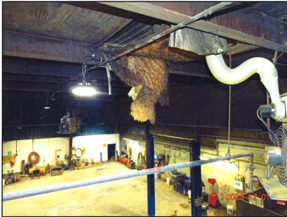
Photo 7: Scattered locations of loose roof insulation.
